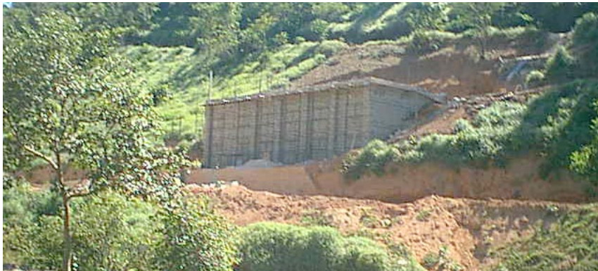
CFR/Minusa Anaerobic digester in Brazil.
